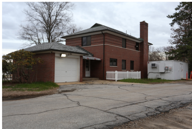
Photo 14: 2022 photograph of the rear of the Manager's Home and its attached garage.
