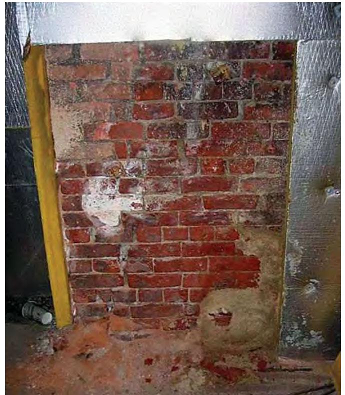
Fig. 21. The interior face of a brick masonry wall shows damage that resulted from the installation of a vapor retardant (foil facing) and thermal insulation. Photo: Simpson Gumpertz & Heger.
