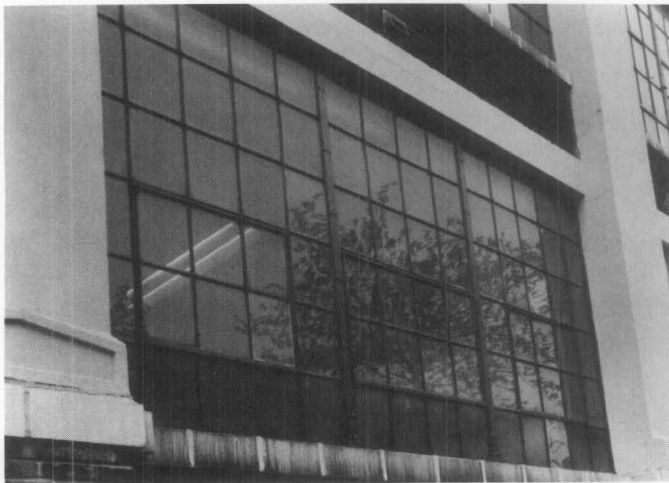
Fig. 10 b. Close-up view of the new replacement steel windows which matched the multi-lighted originals exactly. Photo: Charles Parrott.
