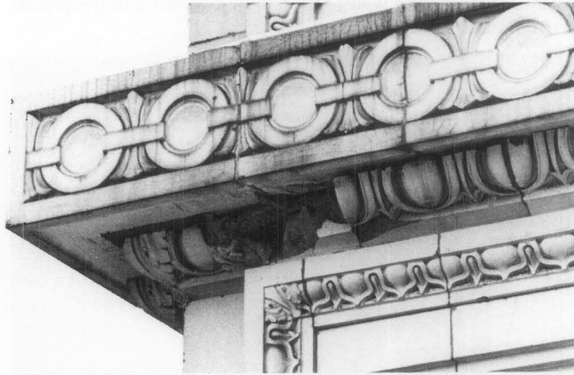
Figure 7. Material Spalling. Excessive expansion of the porous tile body caused by water and freezing temperatures produces major material spalling, a situation often difficult to repair.
