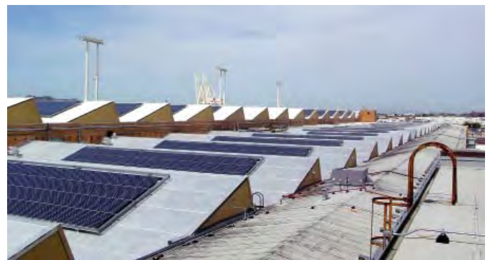
Fig. 23. Solar collectors installed in a compatible manner on low sloping sawtooth monitors. Top Photo: Neil Mishalov, Berkeley, CA.
