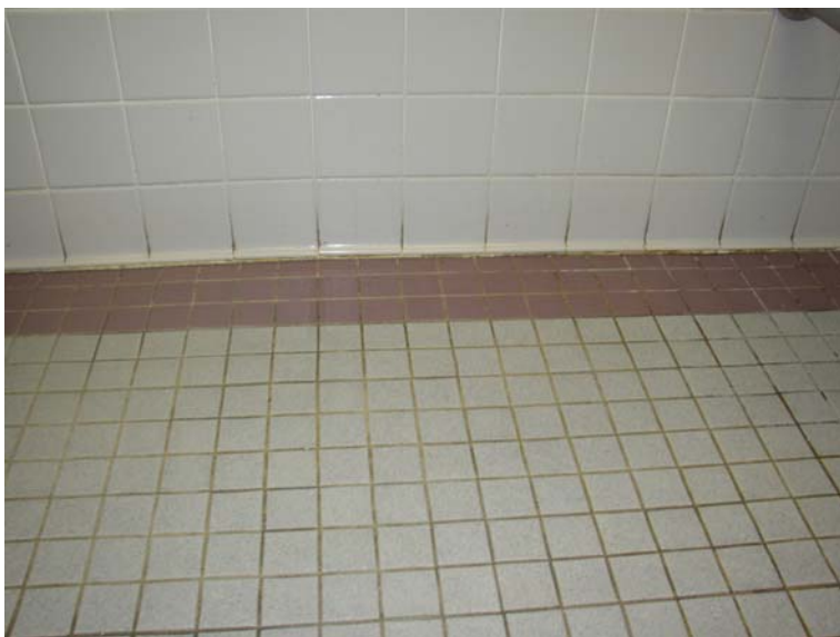
Picture 3 – Public Restroom Floor
