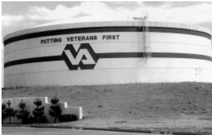
Dallas VAMC's new 3.3 million-gallon thermal storage vessel is one of 92 energy-saving projects VA medical centers have installed or plan to install under Energy Savings Performance Contracts.
